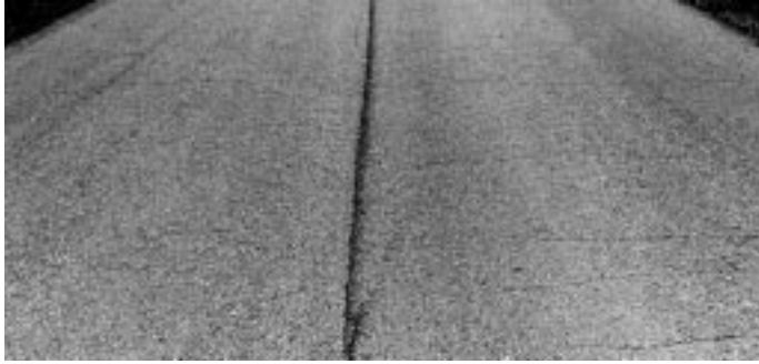
Centerline crack (still tight). ▶
