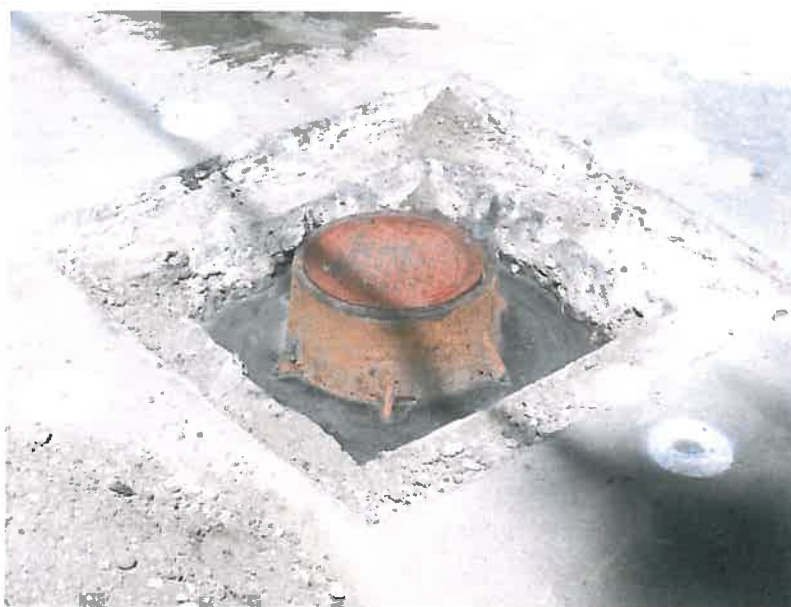
Lids of manhole removed and replaced= 12 lb, manhole frame = 80 lb. Bags of cement = 60 lb.
