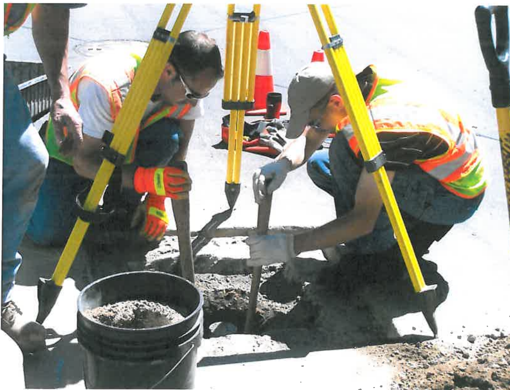
Digging is occasional. Here workers are digging to remove monument. Low squat or kneeling is needed as these are buried in the ground.
