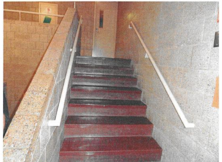
JDC- stairs are up to ADA code.
