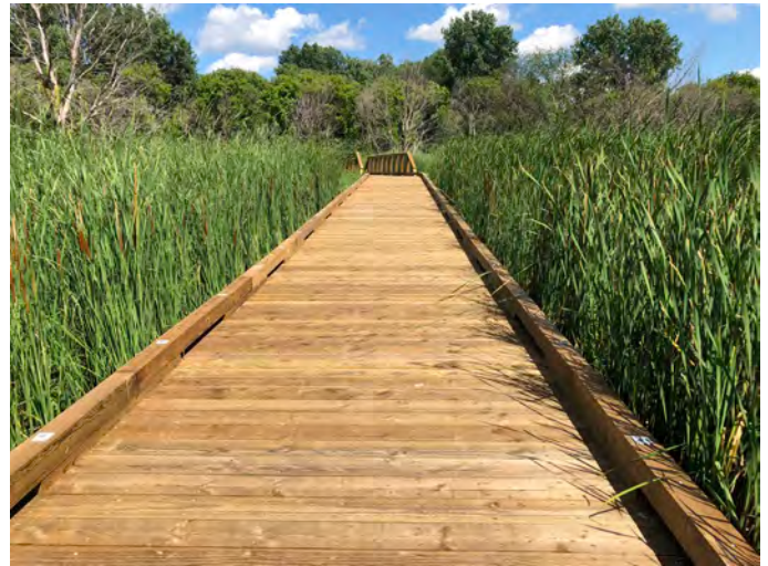
Low boardwalk without railing.
