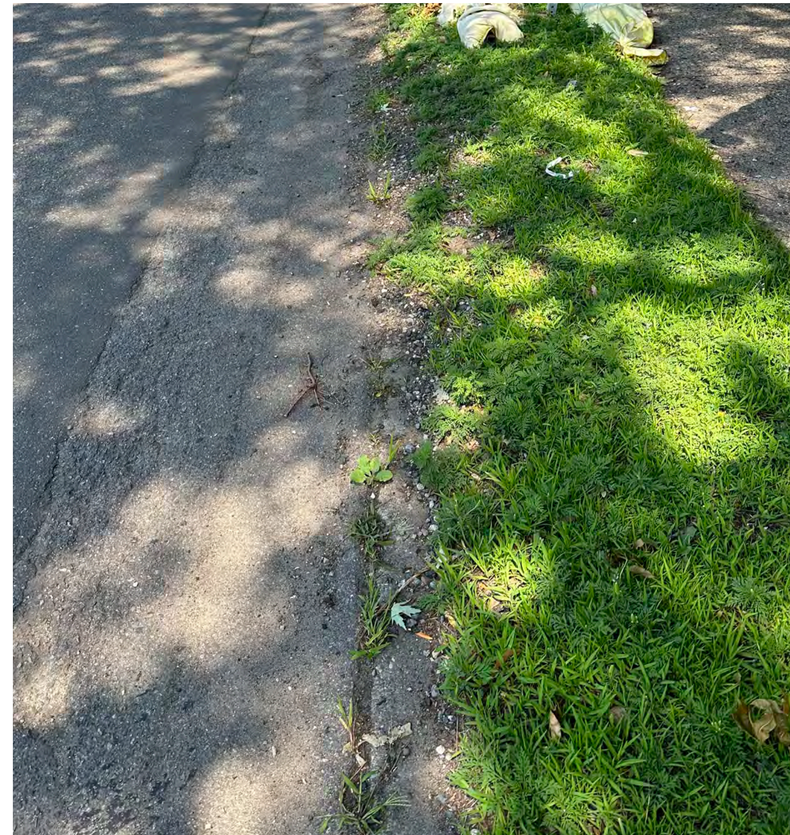
Curb conditions along Dale Street are deteriorated in various locations.
