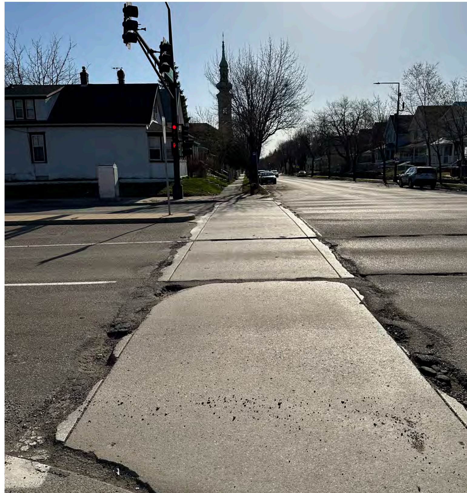
Pavement conditions are very poor and are overdue for resurfacing.
