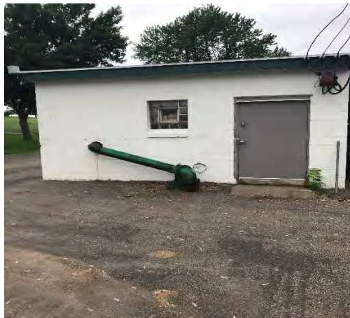
Older deep well pump in good condition
