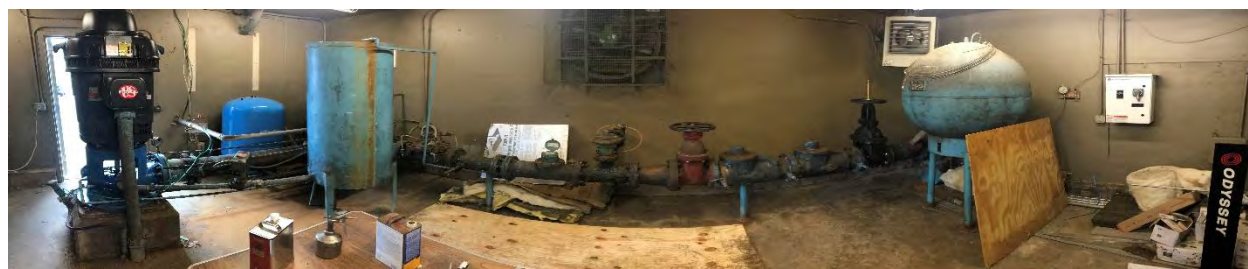
Below – Older Pump House and Controls
