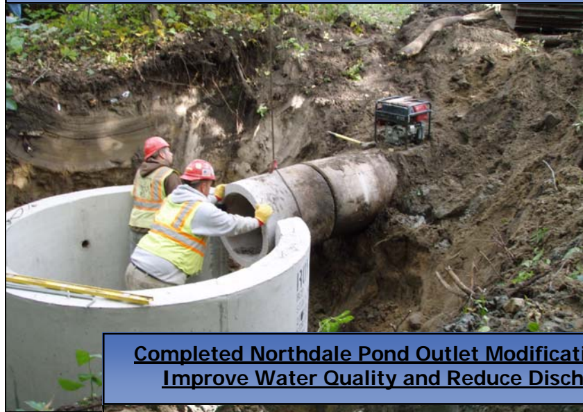
Pond Outlet Retrofit Being Installed on School District Property at Northdale Middle School
