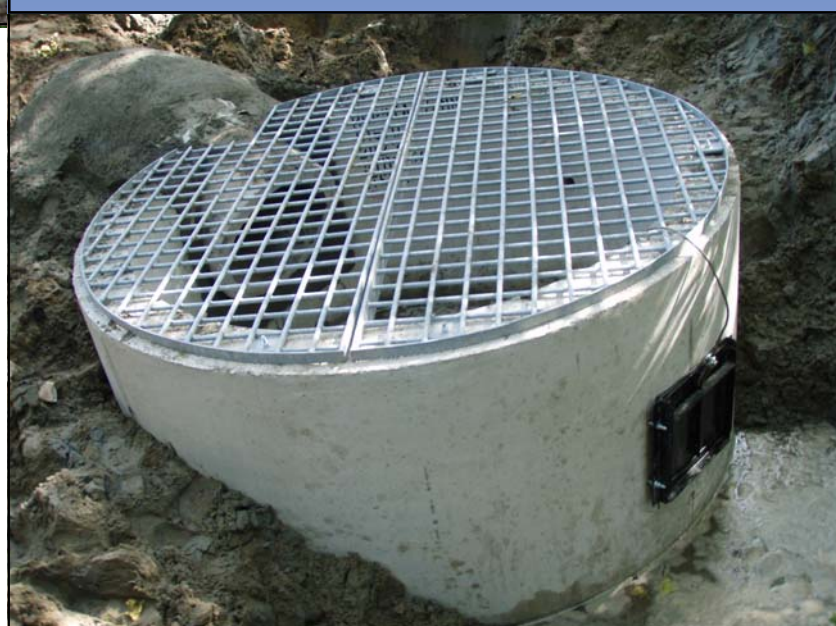
Completed Northdale Pond Outlet Modification Will Improve Water Quality and Reduce Discharge
